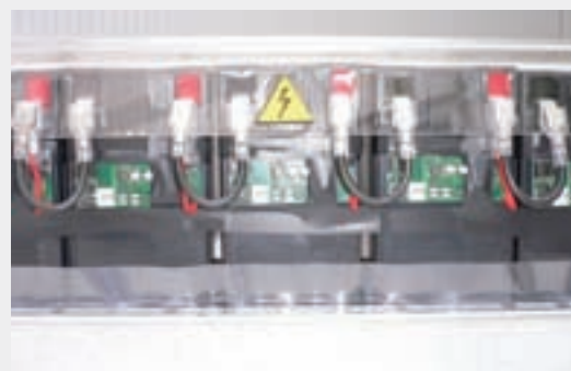
Modules integrated into battery line
