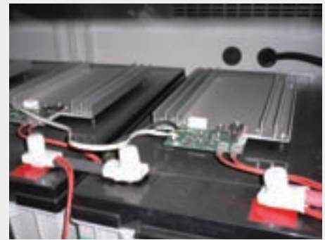
Modules integrated into battery line
