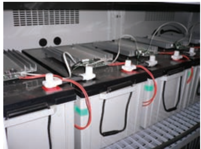
Detail view of single modules. Detection and exchange of defective batteries easily possible.
