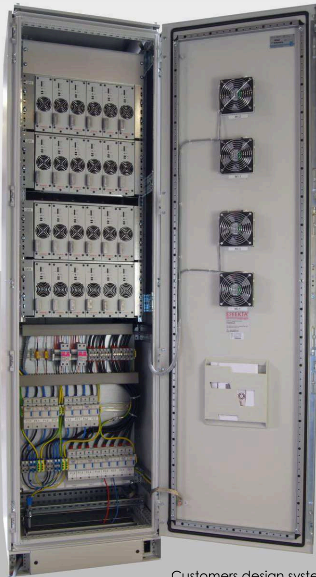
Customers design system (2 x 24.000W redundant)
